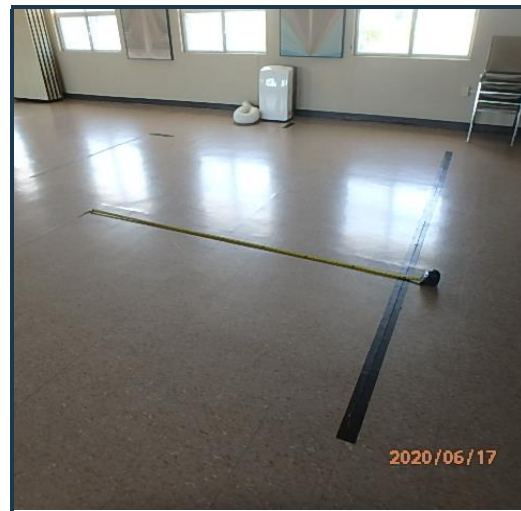
Photo 4: Duct tape over cracks in vinyl flooring
