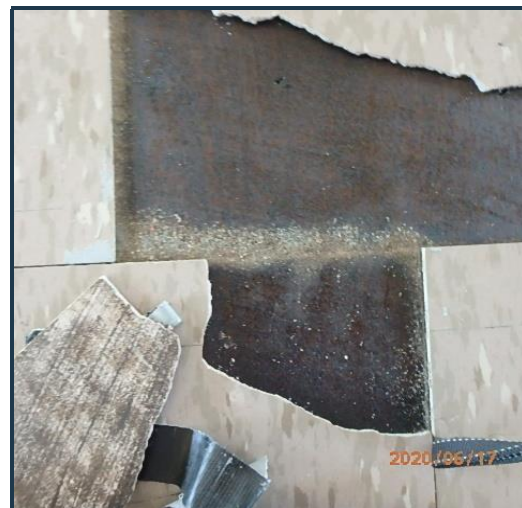
Photo 8: Dirt stain under tile
