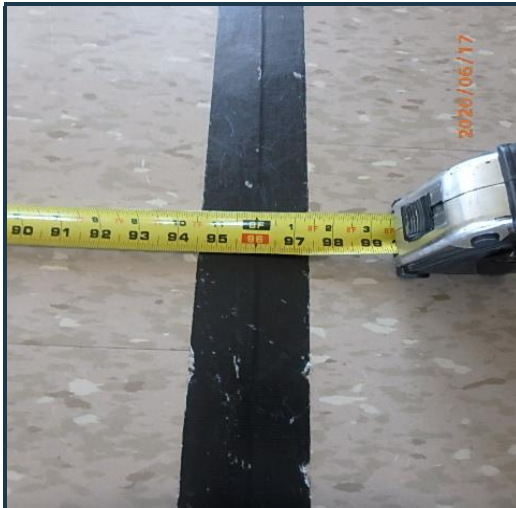
Photo 5: Crack at 8' dimension in subflooring
