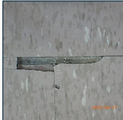
Photo 6: Damaged flooring at subfloor joints
