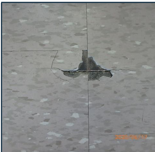
Photo 7: Damaged flooring at subfloor joints
