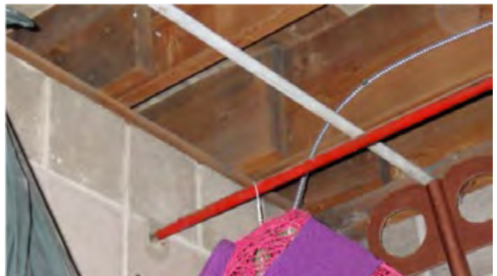
Photo 18 (above): Emergency discharge piping routed through concrete wall of closet used to hang storage item.
