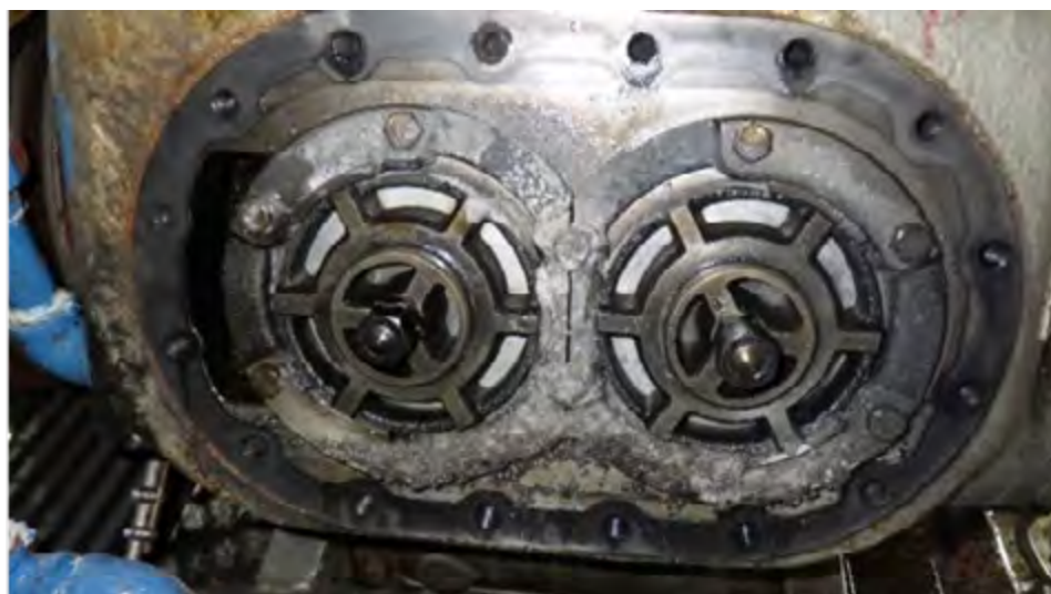
Photo 7: Build-up of salt crystals from brine around lower compressor cylinder heads of compressors #1 and #2.
