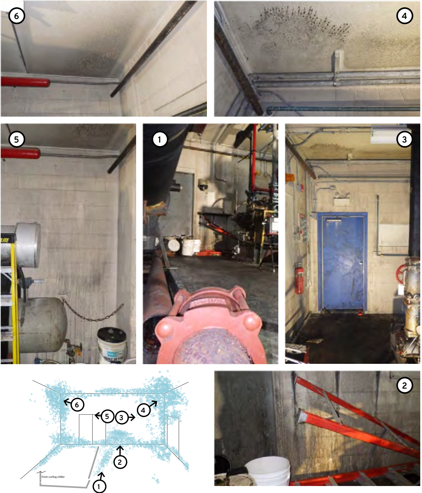
Figure 6: Photos of residue locations on the mechanical room wall. Pattern location is consistent with originating from the separated brine coupling. Samples of the residue tested identified a likely presence of calcium chloride consistent with brine.
