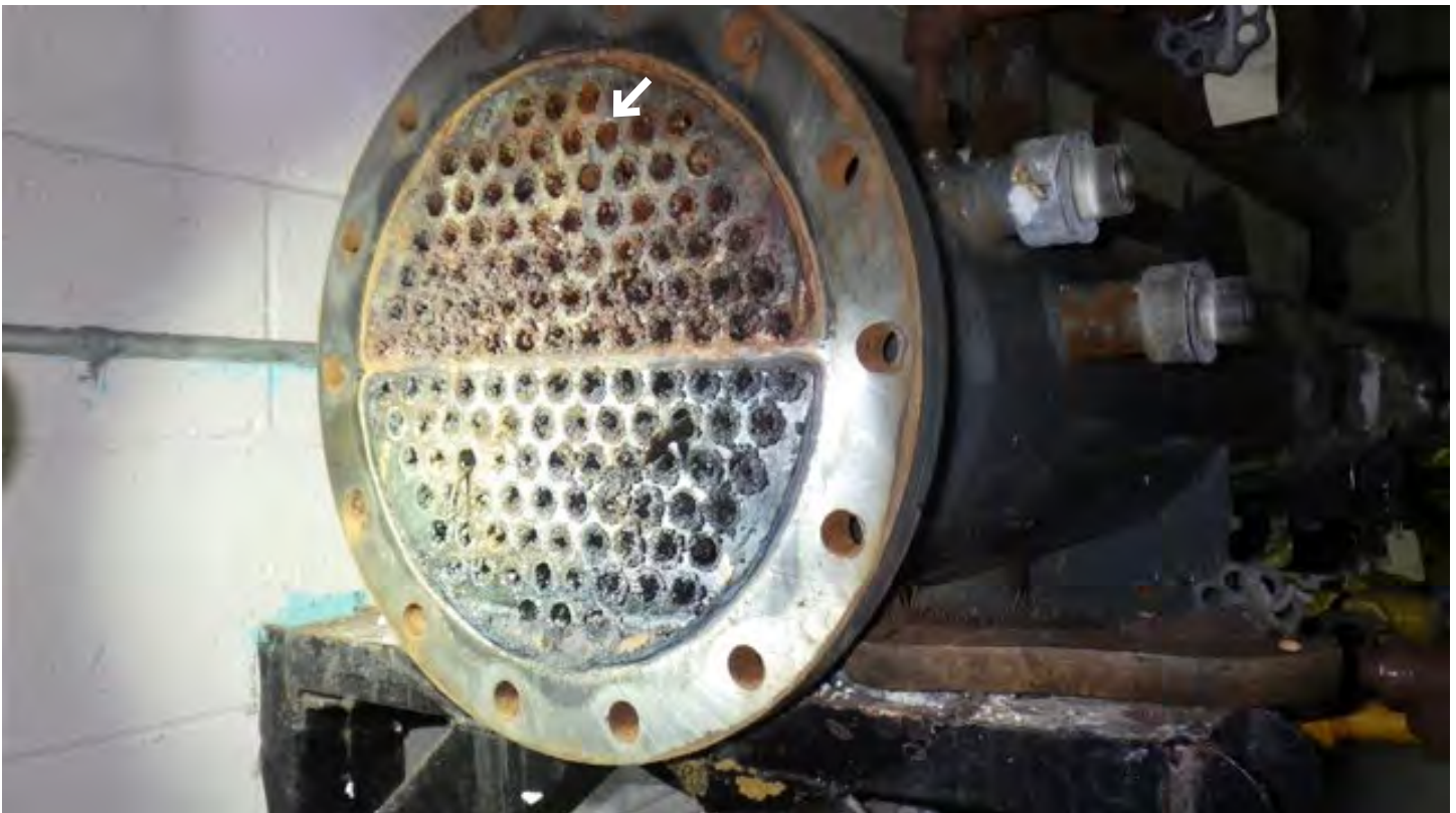
Photo 1: Curling chiller opened showing contamination. The leaking upper tube is identified by the white arrow – second row, third tube from the right side of the photo.
