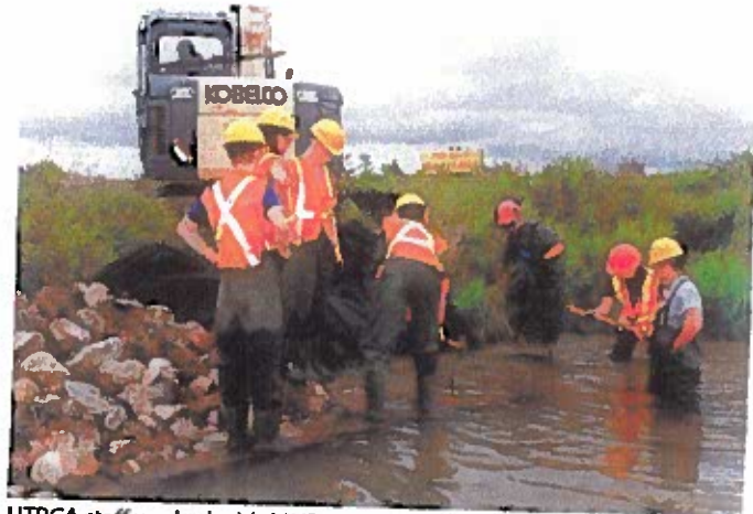
UTRCA staff worked with MNRF Stewardship Youth Rangers to install wooden cover structures along Medway Creek.
