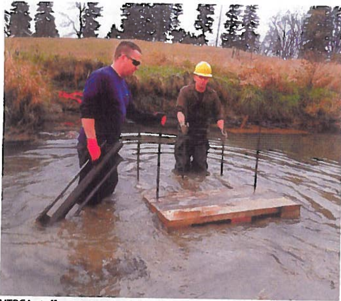
UTRCA staff move an in-stream habitat structure across the stream to install it against the streambank.
