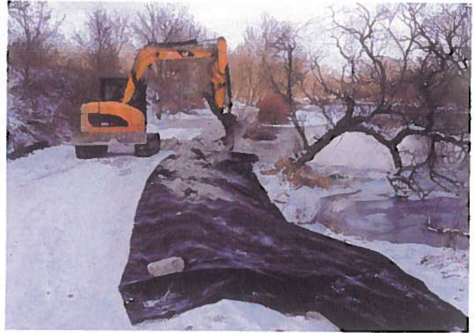
Stone is placed along the river to create a corridor for the trail between the water and the railway embankment.
