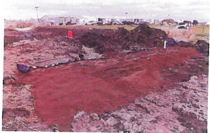
The completed red sand filter.
