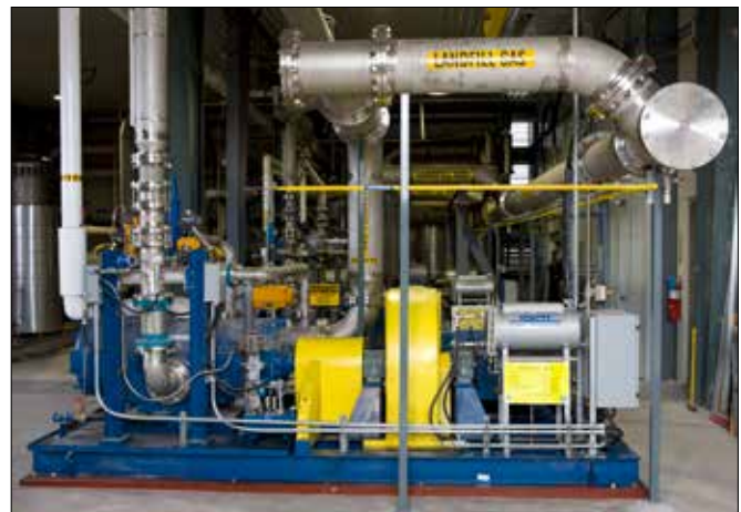
Walker South Landfill - landfill gas utilization infrastructure
