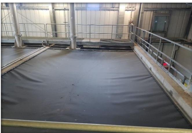
Photo 2: Biological Treatment Process for the Leachate Treatment System
