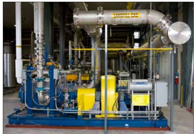
Walker South Landfill - landfill gas utilization infrastructure
