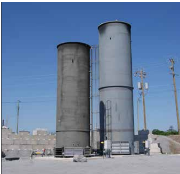
Walker South Landfill - landfill gas flares
