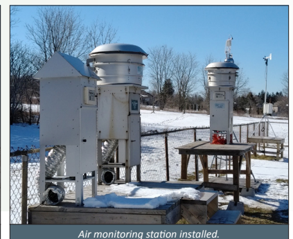
Air monitoring station installed.
