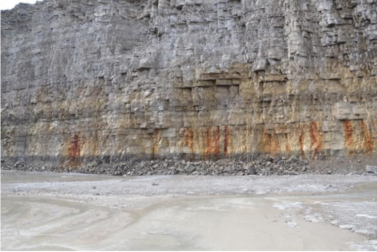
Figure 10. (Top two photos) Staining from the precipitation of iron oxides on the west face of the quarry. The staining shows that most flow into the quarry in this section of the face emanated from a series of point discharges from the same bedding plane.
