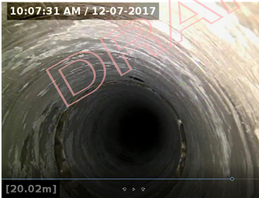
Figure 12. Views looking down BH17-4A in ambient flow conditions. A flow of 5 L/min is flowing from the bedding-plane fracture at a depth of 2.0 m, seen in the top photo, and flowing down the borehole. Additional inflow increases the flow to almost 7 L/min at 20 m, where almost all the flow leaves the borehole.
